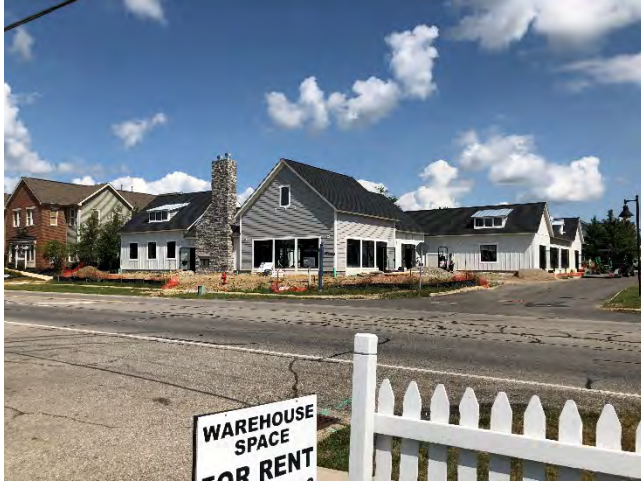
Traditions Retail building under construction located at the northwest corner of West Olentangy and Traditions Way directly east of Touched Home Goods
