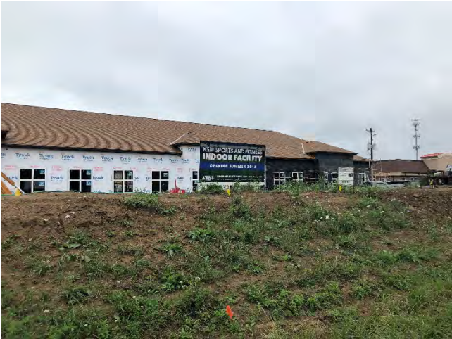
Kids' Sports and Fitness Indoor Facility under construction, located east of the Presidential Parkway shopping center on Sawmill Road
