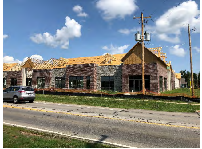
Armita Plaza Shopping Center under construction on the northeast corner of West Olentangy and Traditions Way across from Traditions Retail
