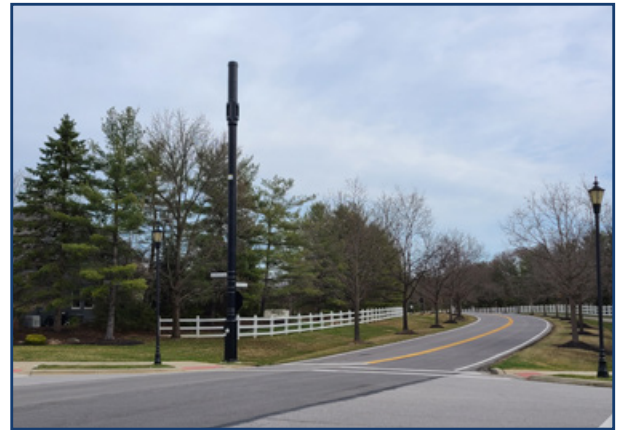
Figure 3.2A--Existing Small Cell Facility at Bennett Parkway and Briarbend Boulevard
