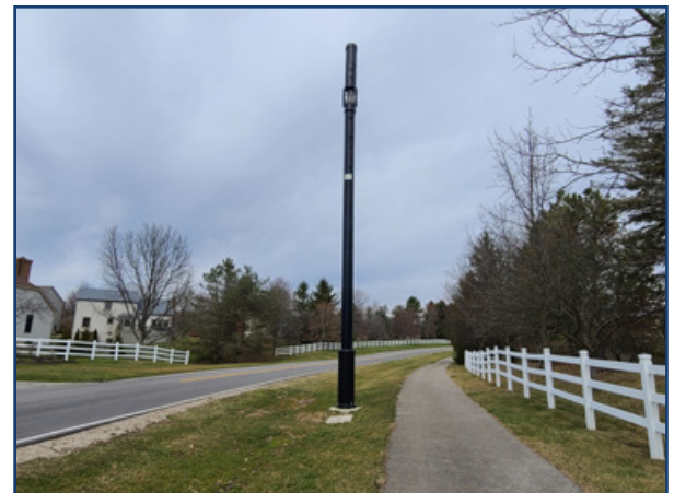
Figure 3.2B--Existing Small Cell Facility at Bennett Parkway and Weatherburn Drive
