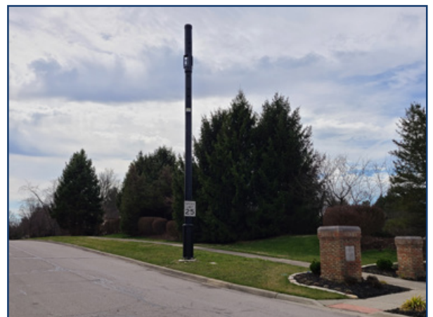
Figure 3.2C--Existing Small Cell Facility at Valley Run Drive and Powell Road
